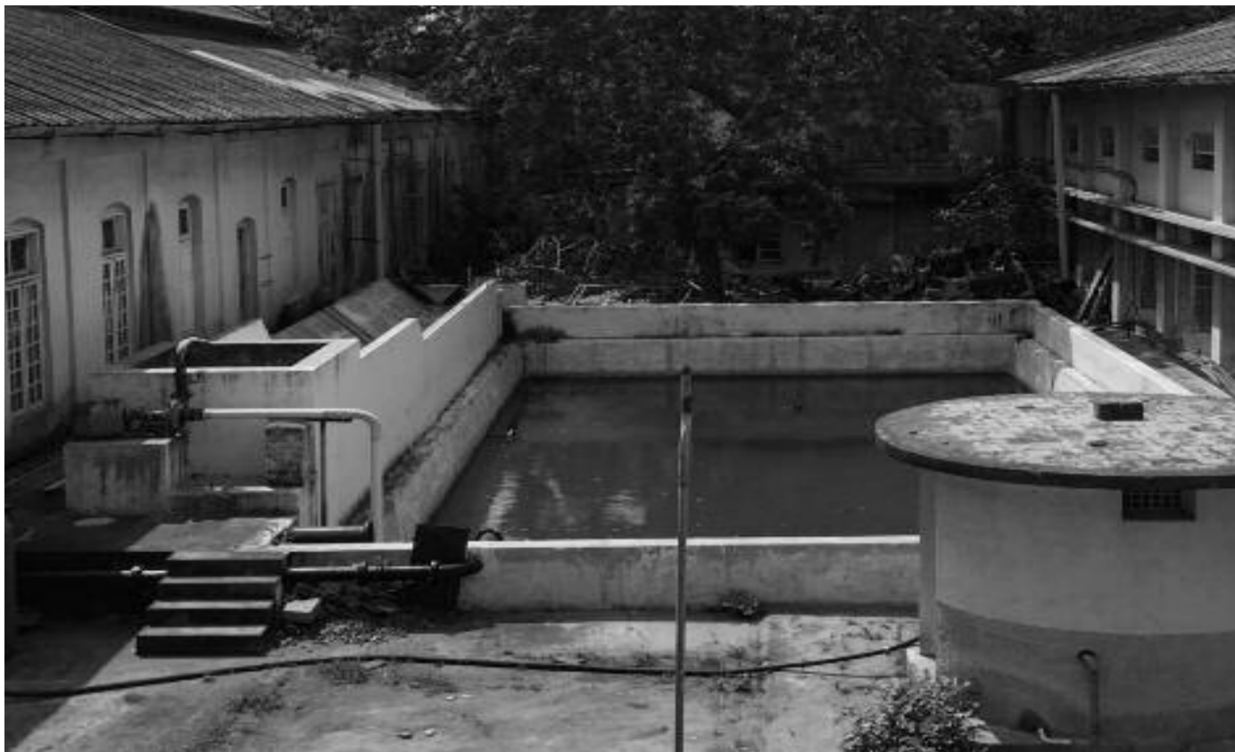
Waste water treatment facility and artificial pond at Anna University
